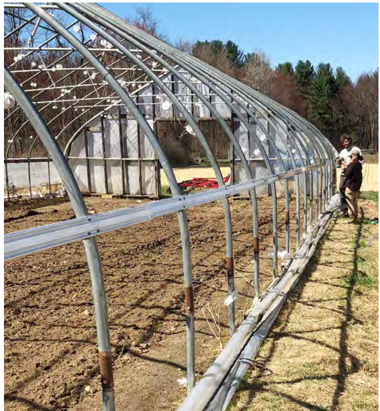
Lia and Will construct new hip walls on the big fieldhouse before re-skinning
